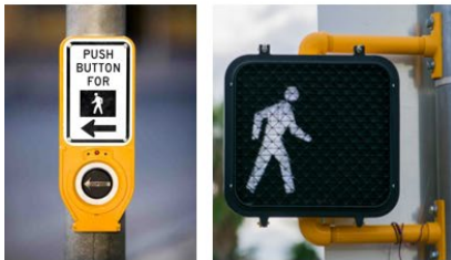
Traffic Signals APS and Peds Signals
